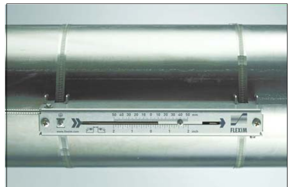
Measurement with transducers mounted by PermaRail
